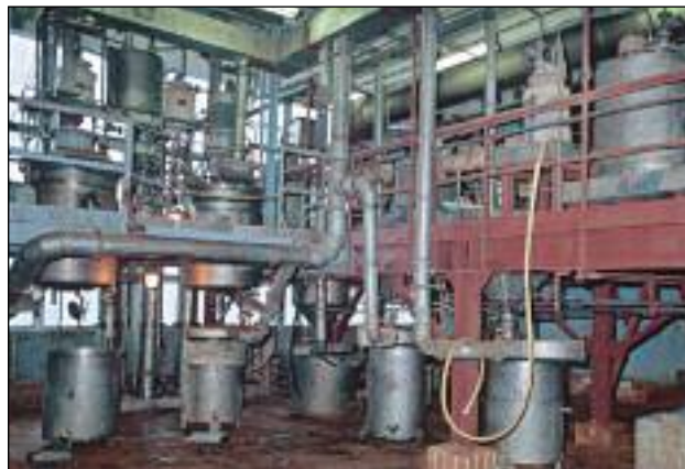
Shelkovsky (Central) opened a new gold refinery in 1996.
