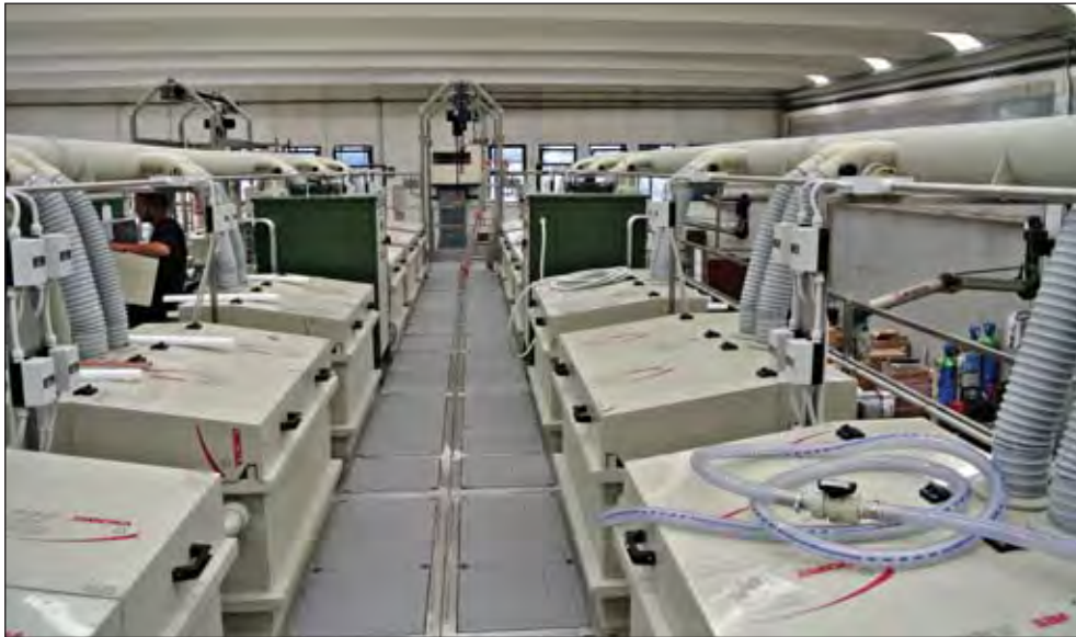
IKOI can design, equip and install, if requested, large or small precious metal refining plants.
